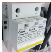
Surge protectors Phase connection on top and earth connection on bottom. Module end of life visual indication.
