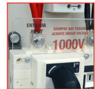
Protection screen This screen prevents direct contact with permanently live parts during maintenance operations
